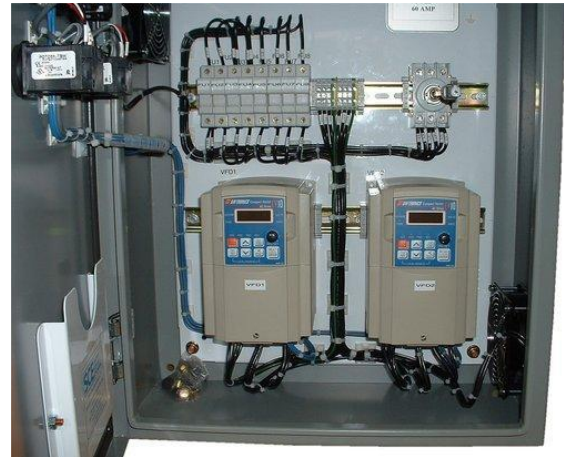
Figure 4 Variable Frequency Drive
